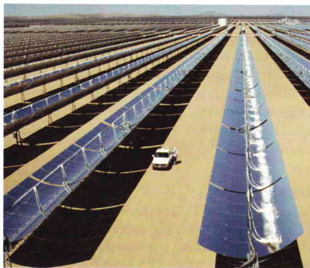
Solar energy power plant in California
